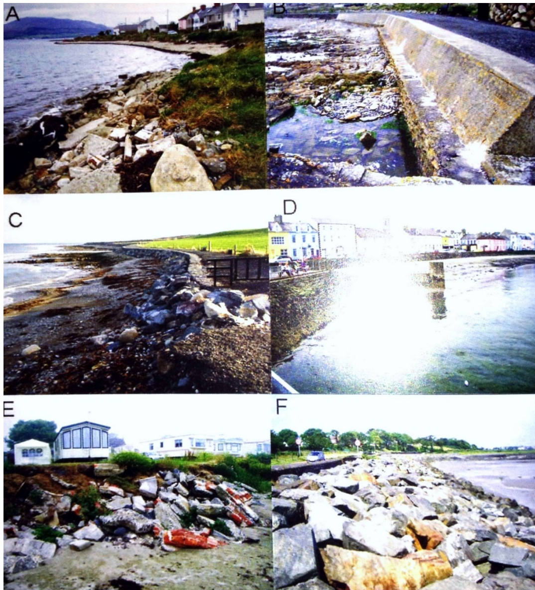
Fig. 3.10. A collage of typical coastal protection structures in Ireland. a) rubble protecting private houses b) precast concrete structure protecting footpath c) gabions protecting footpath d) urban seafront with several generations of walls e) rubble protecting caravan site f) rock armour protecting coastal roads. (Redrawn from: Pranzini E., and Williams A., “Coastal Erosion and Protection in Europe”, 2013)
