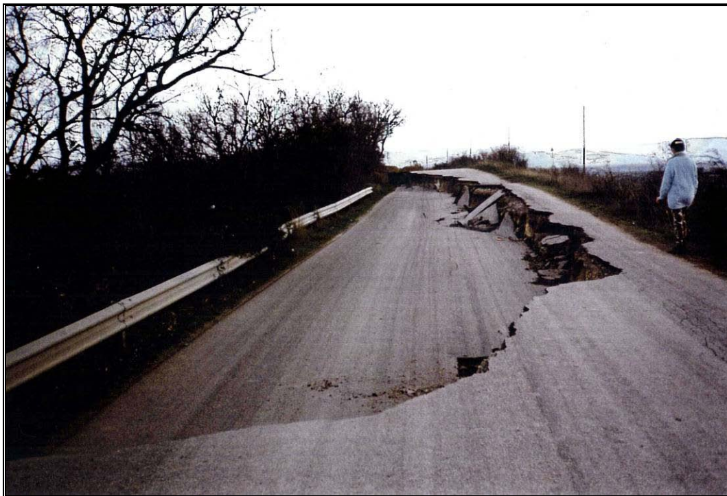
Figure 2: "Vaccareggia", crack on the road at the slide top boundary.
