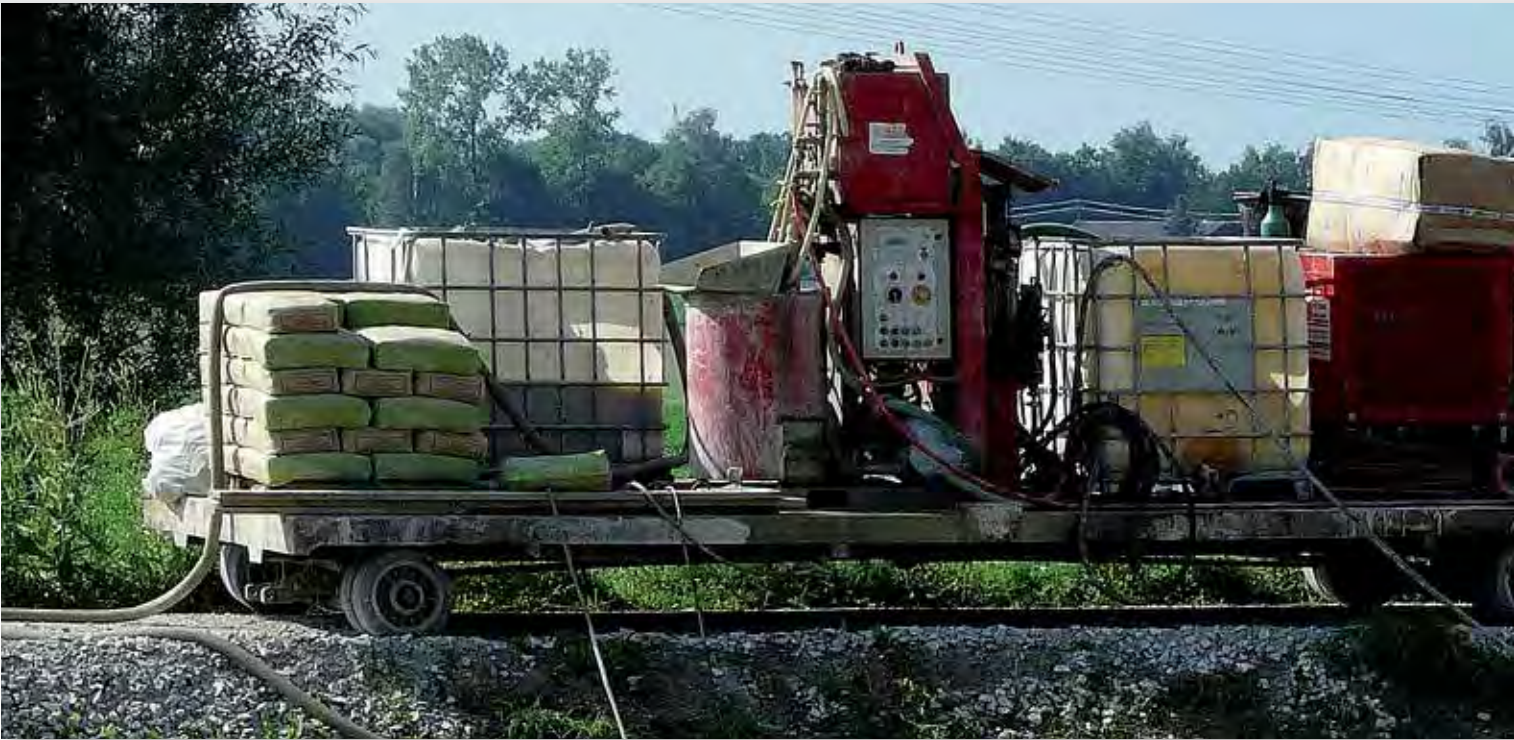
A typical site setup consisting of a grouting unit and a drilling rig mounted on construction plant.
