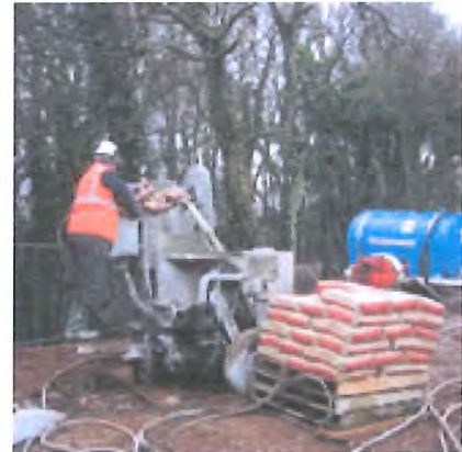
Grout pump with colloidal mixing unit
